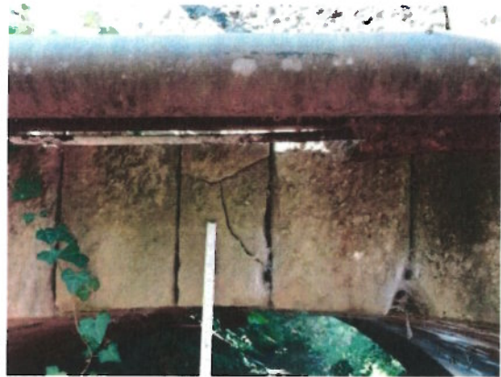
17H-BOGENSTEIN RE GERISSEN 33
